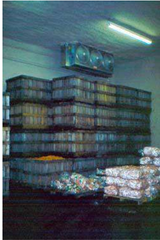
Fig. View of room cooling
